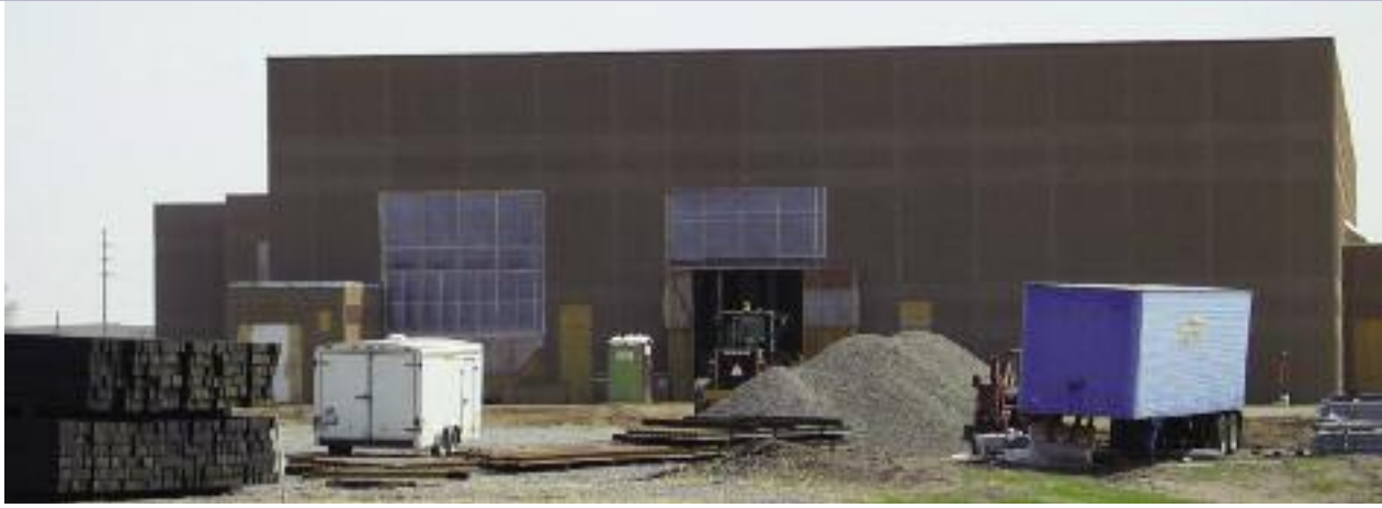
Northstar Maintenance Facility — Big Lake
